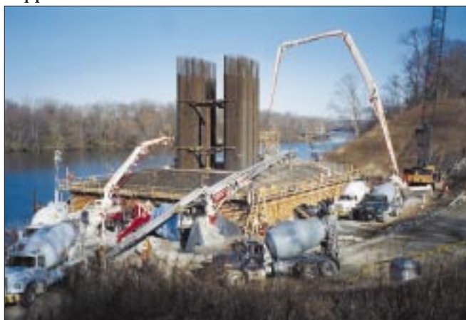
The support structures for the bridge and approach ramps were poured in place, and the size and complexity of these mass-concrete structures required careful management of temperature during the curing process.
